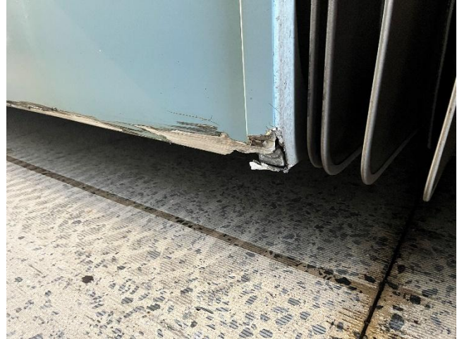
Figure 5.10: Example of Flash vehicle body panel damage immediately behind the articulating bellows. The damage is caused by the outward sweep of the rear body skirt during sharp turns adjacent to stations. Designers should always be mindful of vehicle-station compatibility and approach/departure geometry when modifying BRT stations or procuring new BRT fleets.
